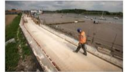
Figure 6. Durability of Cemfree was key to being used for tidal sea defence in Woodbridge, Suffolk.
