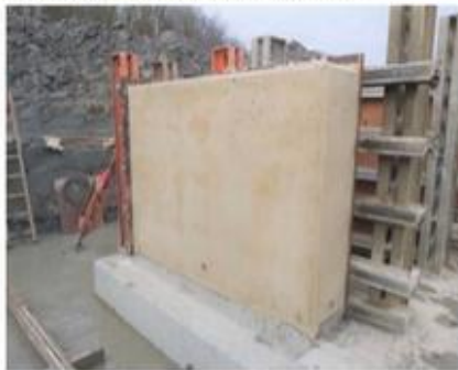
Figure 5. Formwork being stripped on Cemfree wall prior to use on A14 major roadway in Cambridgeshire later this year.
